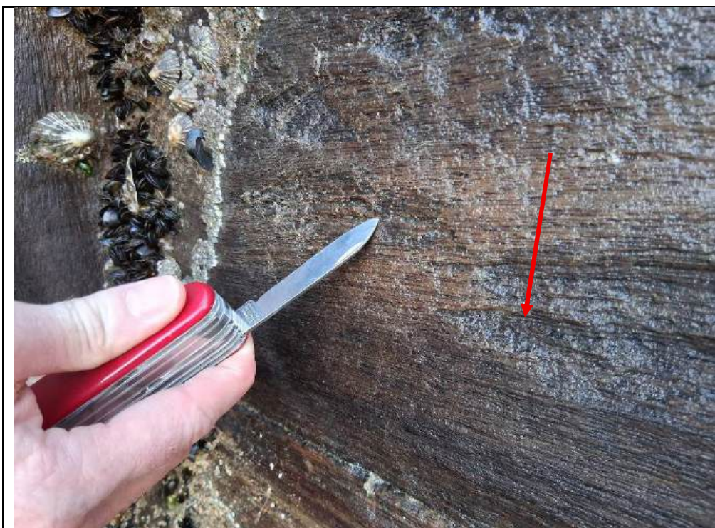
Plate 8 - Groyne C36. Erosion of the face of a plank in the intertidal zone. The plank has suffered some erosion as indicated by the knife. The arrow shows a combination of grazing behaviour and subsequent erosion. Visual assessment rating '2'.
