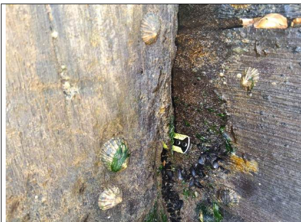
Plate 14 - Groyne C36. A close-up image of gribble attack showing the typical appearance of the exposed galleries in the backwash zone adjacent to the landward face of pile 5. Note the extension of the measuring tape through a gap between the pile and plank indicating loss of section of both, caused predominantly by gribble attack and exacerbated by erosion. Although localised, the visual assessment rating for the plank is '3'.
