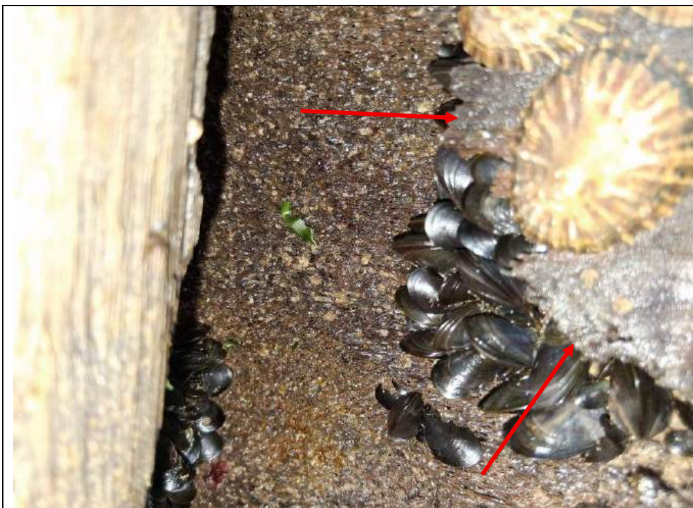
Plate 12 - Groyne C36. An close-up image of gribble attack showing the typical appearance of the exposed galleries at the boundary of the surface of the plank and the 'gribble zone' (indicated). The visual assessment rating is '3'.
