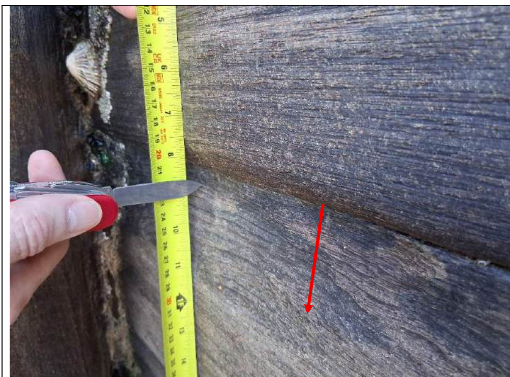
Plate 9 - Groyne C36. Typical 'scalloped' appearance of a plank caused by backwash of sediment as indicated by the knife. The faint pitted appearance (indicated) suggests erosion has exposed and eroded gribble galleries. The visual assessment rating is '2'.
