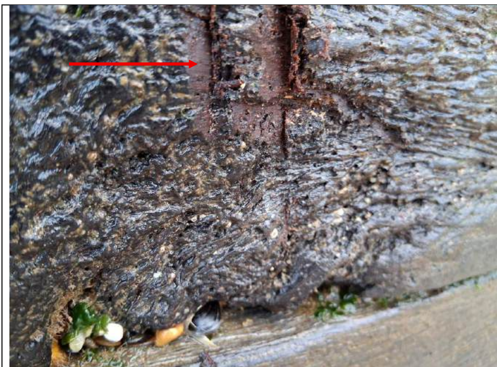
Plate 6 - Groyne C36. Typical pattern consistent with gribble attack showing galleries just below the surface that are eroded away by wave action. Striking the surface of the plank shows the galleries are shallow (indicated). The visual assessment rating for this plank ( Table 5.1 ) was '2', although the image focusses on a small part of the plank.
