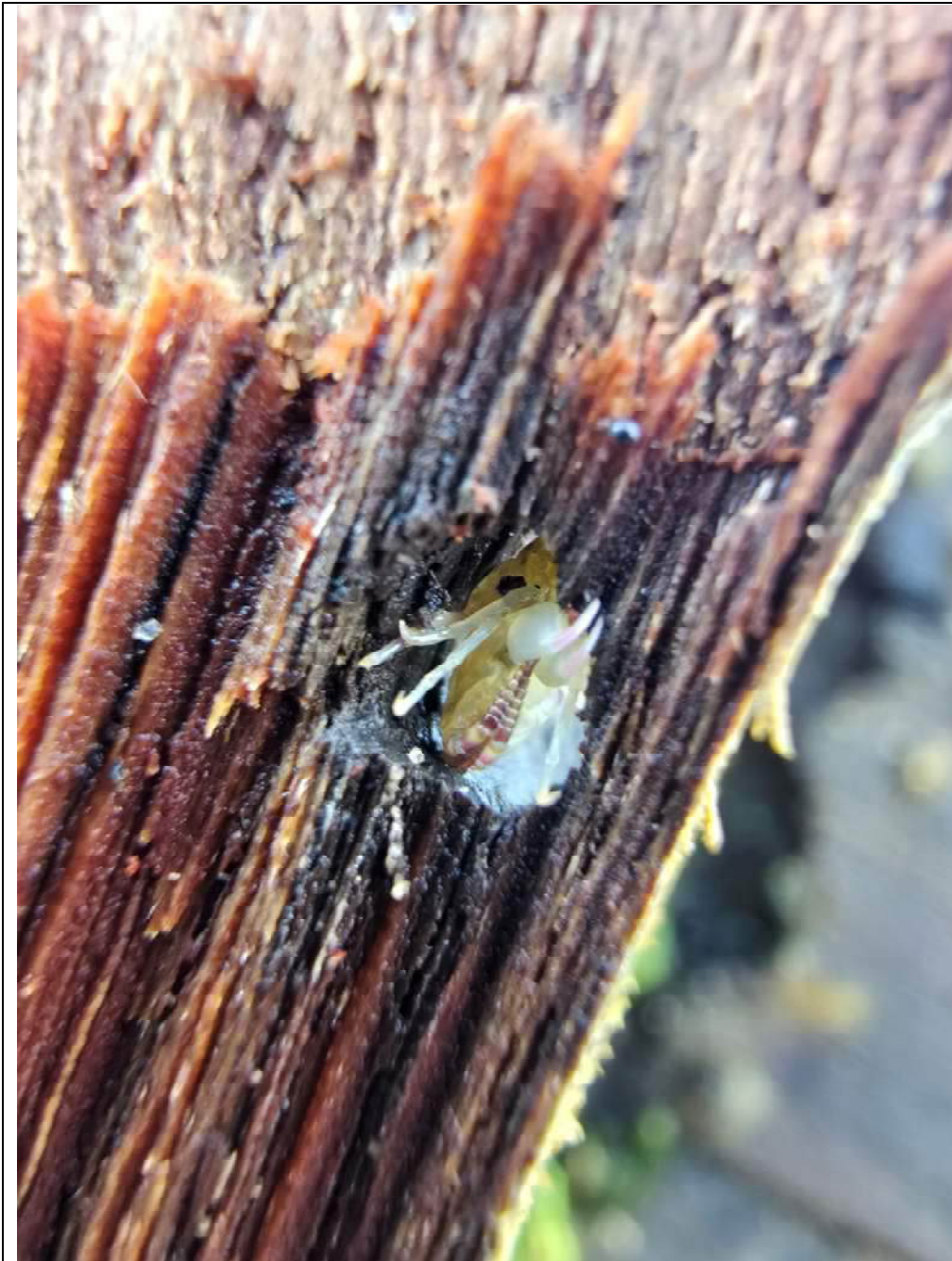
Plate 22 - Groyne C36, pile 5. Breaking open the timber exposed an animal dwelling in the tunnel, most likely a gammaridean amphipod, a small shrimp-like crustacean.
