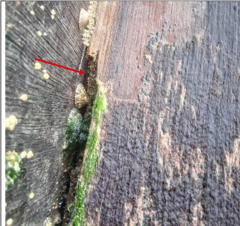
Plate 28 - Groyne 37. Gribble attack at the edge of a greenheart pile on the seaward face. The damage is limited to the paler timber, which may be less resistant sapwood. The localised nature of the damage and minor loss of section at the edge of the pile results in a visual assessment rating of '2'.
