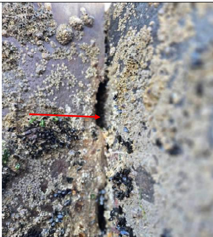
Plate 31 - Groyne 37. Slight loss of section at the edge of pile 1 on the landward face (indicated) caused by gribble attack. There was no equivalent damage on the adjacent ekki planks. The localised nature of the damage and minor loss of section at the edge of the pile results in a visual assessment rating of '2'.
