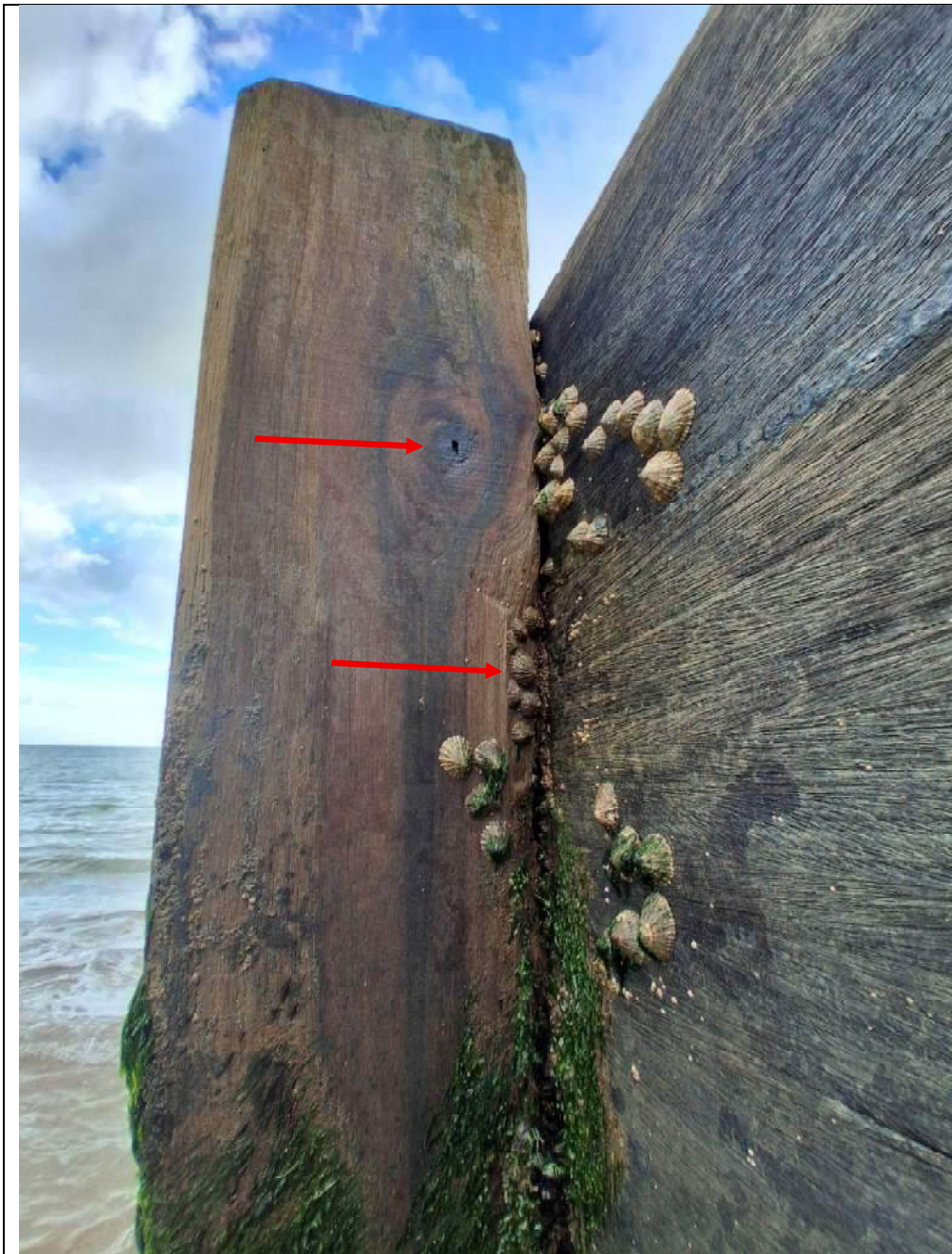
Plate 27 - Groyne 37. Contrast between a greenheart pile and ekki planking. The pale edge of the greenheart coincident with the ekki planks appears to be slightly eroded and may be a sign of less durable sapwood which can be present on large cross section greenheart piles. The knot (indicated) in the darker heartwood causing distortion in the colouration of the pile reinforces the assertion that the paler wood comprises sapwood. There has been some erosion of the landward face as indicated by the barnacles lodged onto the timber (indicated).
