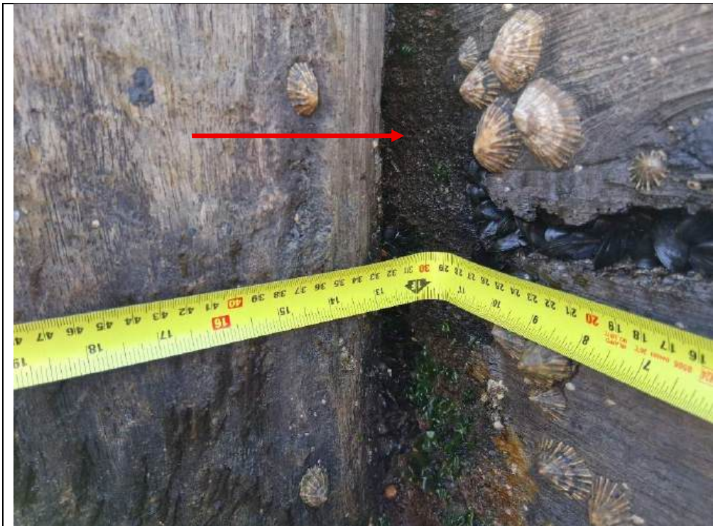
Plate 11 - Groyne C36. An example of erosion observed on the landward face of a pile caused by backwash of sediment abrading the pile surface. This action can create refugia for gribble, which in this case (indicated) has colonised a sheltered part of the groyne and started to attack the plank. The visual assessment rating is '3'.
