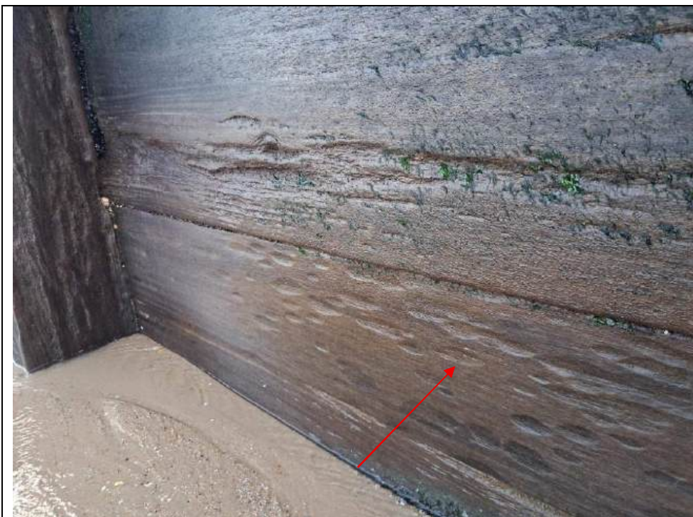
Plate 16 - Groyne C36. A wider-angle view of Plate 15 illustrating section loss caused by a combination of gribble attack and erosion (visual assessment rating '2') and an unusual pattern of erosion in the plank below (indicated), which has not been caused by gribble attack. This pattern may have been caused by erosion of pockets of lower density timber or of soft rot pockets. This image shows the variable nature of basralocus.
