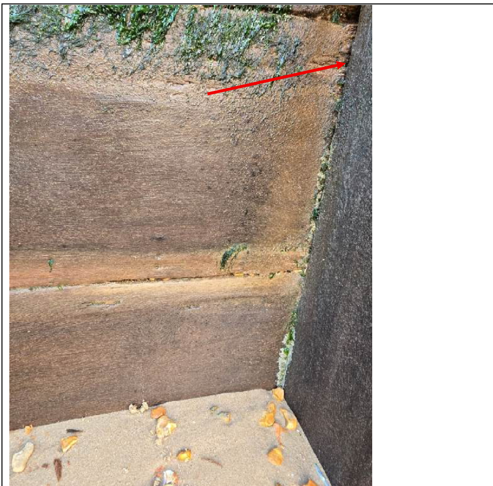
Plate 42 - Groyne 30. Gribble attack observed at the edge of a plank adjacent to a pile on the seaward elevation (indicated). The localised nature of the damage and minor loss of section at the edge of the plank results in a visual assessment rating of '2'.
