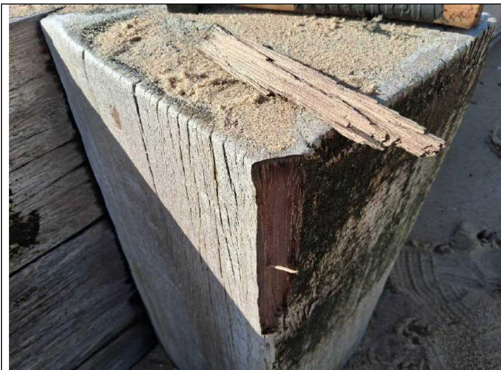
Plate 3 - Groyne 36: Removal of pile edge to examine the timber characteristics to confirm the piles comprised basralocus. This was also confirmed by measuring the cross section, which exceeded the standard 300 x 300 mm pile section for greenheart piles. A larger 330 x 330 mm cross section was selected to counter the reduction in strength of basralocus (D50 est.) when compared in greenheart (D70).
