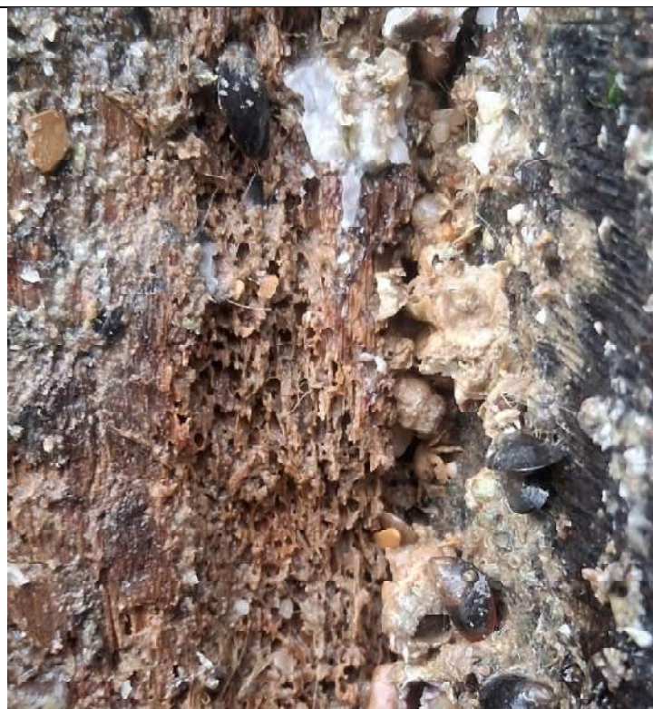
Plate 30 - Groyne 37. Close-up image of gribble attack at the edge of a greenheart pile on the more sheltered landward face. Note the contrast between the greenheart and darker ekki, which has not been attacked by gribble. The localised damage and minor loss of section at the edge of the pile results in a visual assessment rating of '2'
