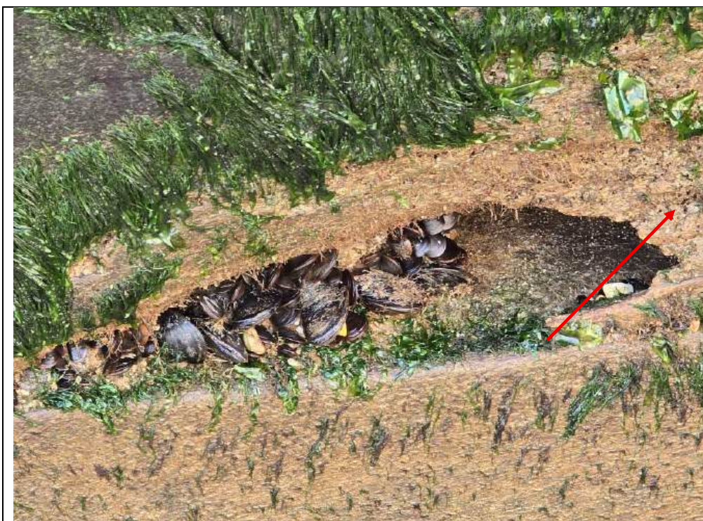
Plate 40 - Groyne 30. Localised voiding of a plank. The most likely explanation is gribble attack of a softer part of a plank, which may have been caused by a pocket of incipient decay in the tree. Some gribble colonisation was observed (indicated). The localised nature of the damage and minor loss of section at the edge of the plank results in a visual assessment rating of '3'.
