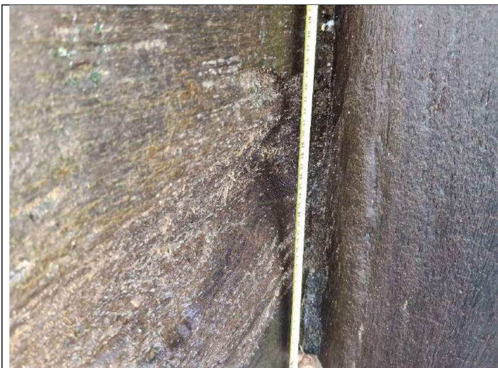
Plate 17 - Groyne C36: Loss of section of a plank adjacent to the seaward face of a pile. This loss has been caused by a combination of gribble attack and subsequent erosion.
