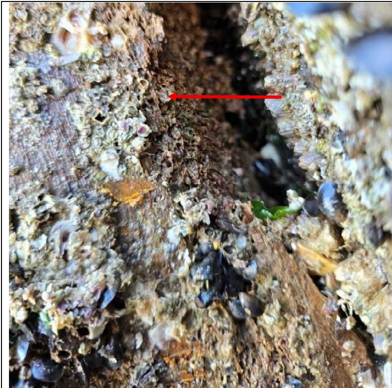
Plate 32 - Groyne 37. Galleries characteristic of gribble attack on pile 1 (indicated).
