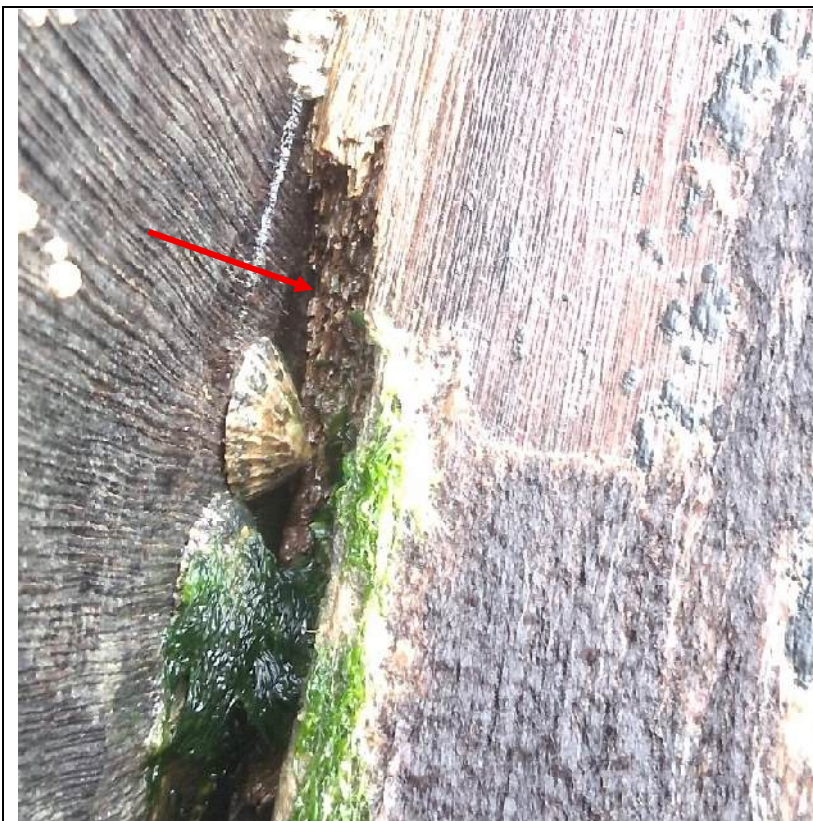
Plate 29 - Groyne 37. A close-up image of Plate 28 showing the gribble favouring to colonise and damage the greenheart (indicated) and not attacking the ekki.
