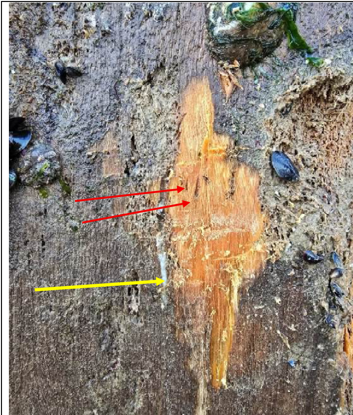
Plate 38 - Groyne 37, pile 4. The yellow arrow indicates a shipworm tunnel. The red arrows indicate part-formed tunnels as a consequence of the larvae failing to lodge into the timber. The localised nature of the damage and minor loss of section at the edge of the pile results in a visual assessment rating of '2'.
