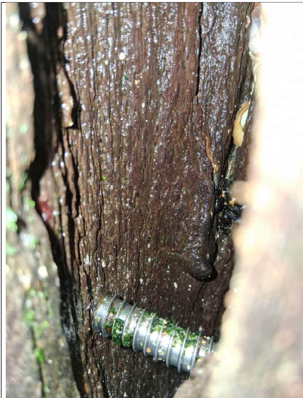
Plate 19 - Groyne C36. Close up of the cavity of pile 9 shown in Plate 18 illustrating the 'hollowing out' of the pile.
