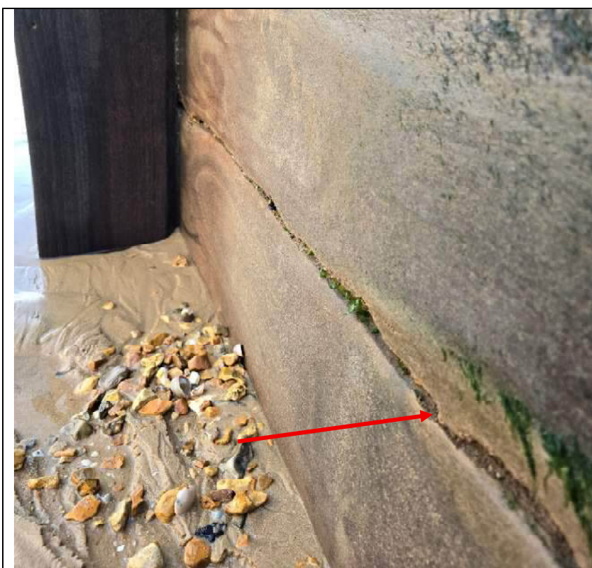
Plate 41 - Groyne 30. Gribble attack observed at the edge of a plank (indicated). The localised nature of the damage and minor loss of section at the edge of the plank results in a visual assessment rating of '2'.
