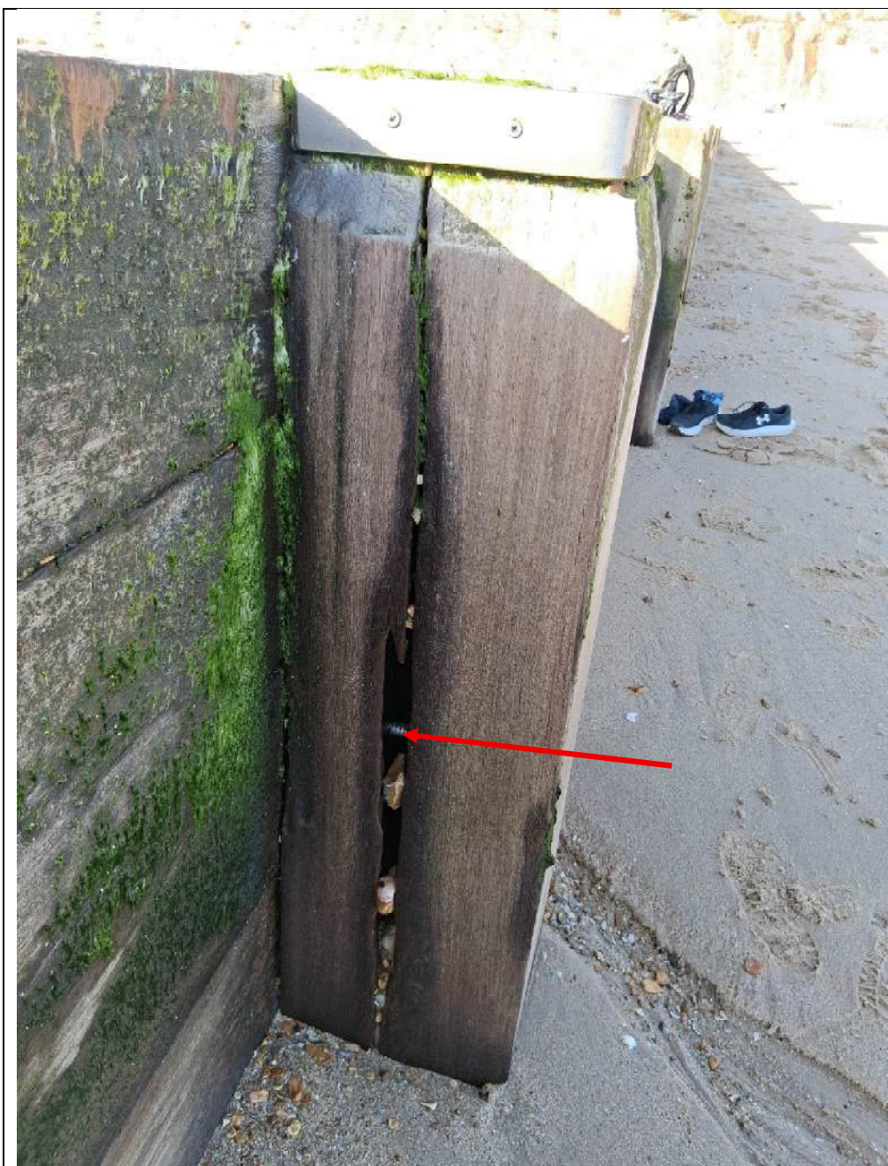
Plate 18 - Groyne C36. Pile 9. Substantial internal 'hollowing out' damage to a basralocus pile caused by gribble attack. This pile is at risk of failure; visual assessment rating '4'.
