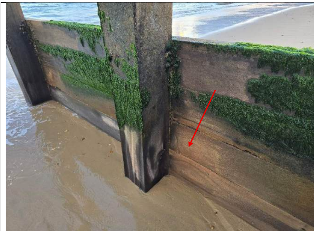
Plate 39 - Groyne 30. General appearance of the greenheart piles and planks with some minor scalloping observed on the down-drift elevation (indicated).
