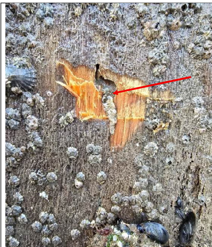
Plate 36 - Groyne 37. Scraping away the surface layer of timber on pile 4 around a suspected shipworm siphon revealed the calcareous lined tunnel of a juvenile shipworm (indicated).
