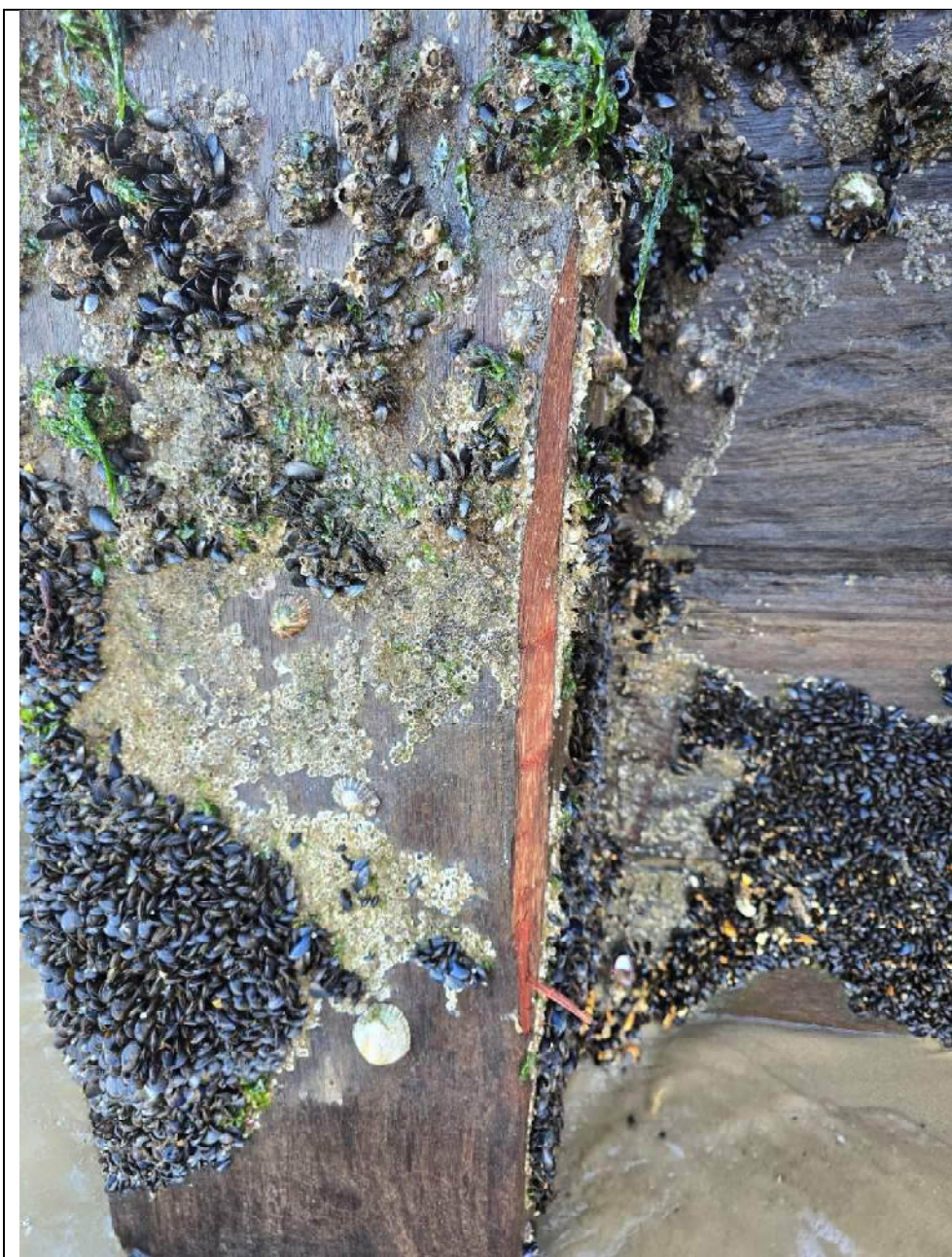
Plate 5 - Groyne 36. Pile 2. No evidence of shipworm.
