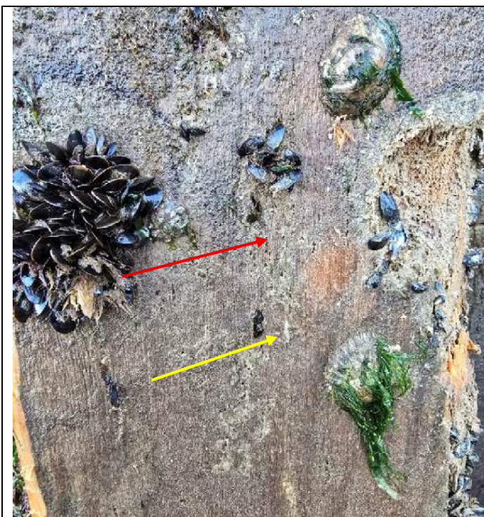
Plate 37 - Groyne 37, pile 4. Suspected shipworm siphons (indicated) and the likely exposure of the calcareous lining of a shipworm tunnel (yellow arrow). The localised nature of the damage and minor loss of section at the edge of the pile results in a visual assessment rating of '2'.
