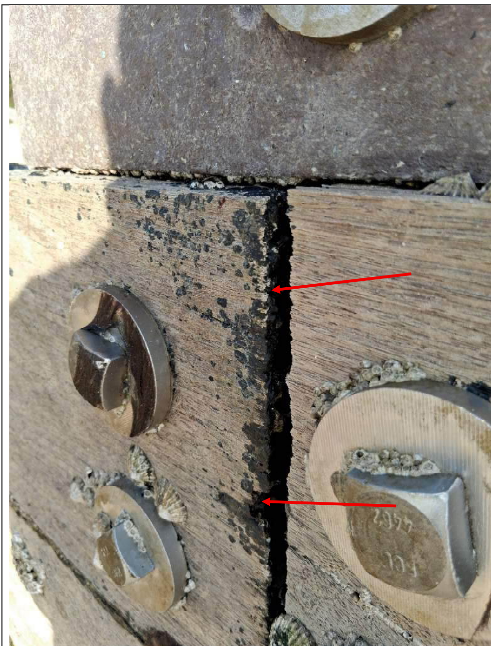
Plate 23 - Groyne C36. Evidence of gribble damage to the end grain of adjacent planks (indicated) on the updrift face of the groyne where the planks are fixed to pile 5. Damage was typically seen on the more sheltered downdrift face. The loss of section within the plank results in a visual assessment rating of '4'.
