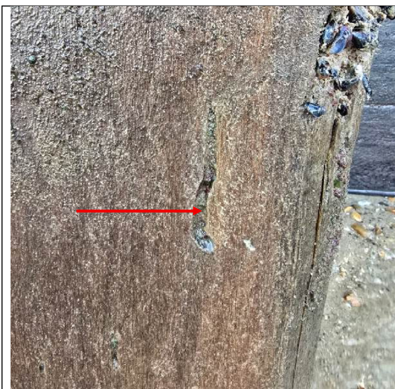
Plate 35 - Groyne 37. Shipworm tunnel exposed by abrasion of the surface of pile 4.
