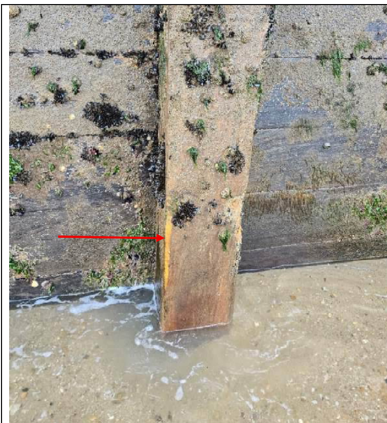
Plate 33 - Groyne 37. An example of assessment for shipworm attack by removing the edge (indicated) of pile 4 to a length of ca. 500 mm in order to expose shipworm tunnels (photograph taken whilst work was in progress).
