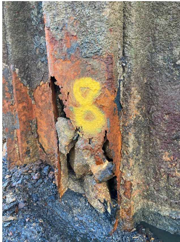
Figure 3-1 Serious holing caused by ALWC at Weymouth Harbour Wall C (captured 2 nd February 2022).
