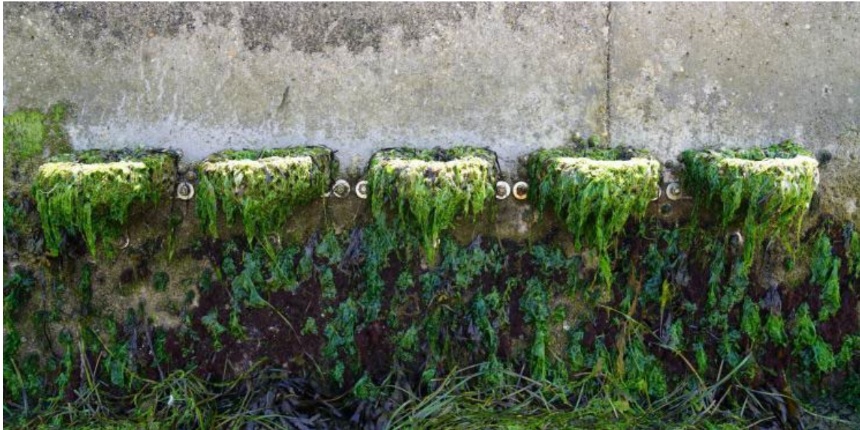
Figure 4-1 Artificial rockpools constructed on a vertical wall comprised of smooth concrete (Channel Manche, 2022b).
